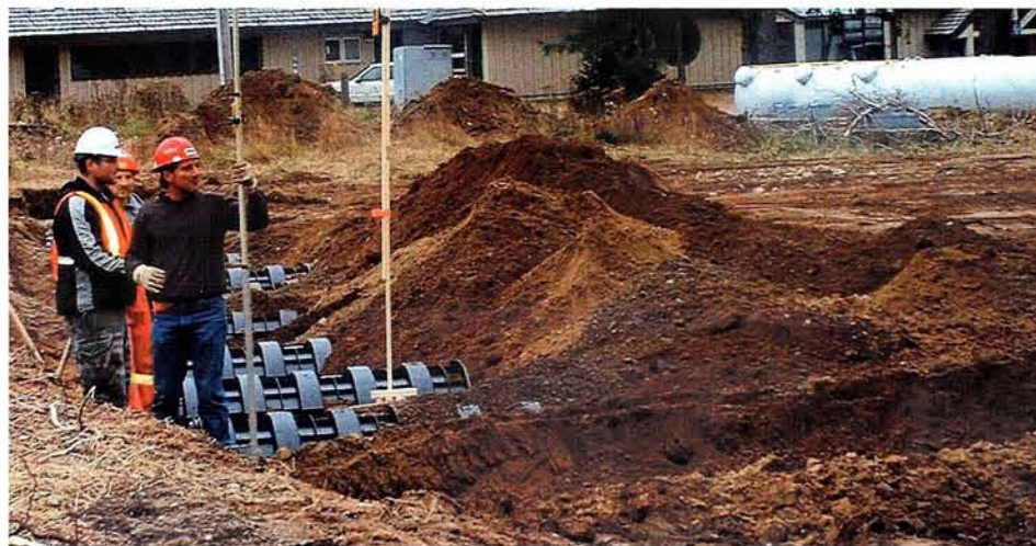
Because of the mountain location and lack of available suitable land, chambers were used for the new disposal field.
